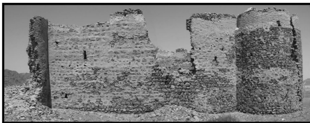
Plate (2-c): The S-E façade destructions.
